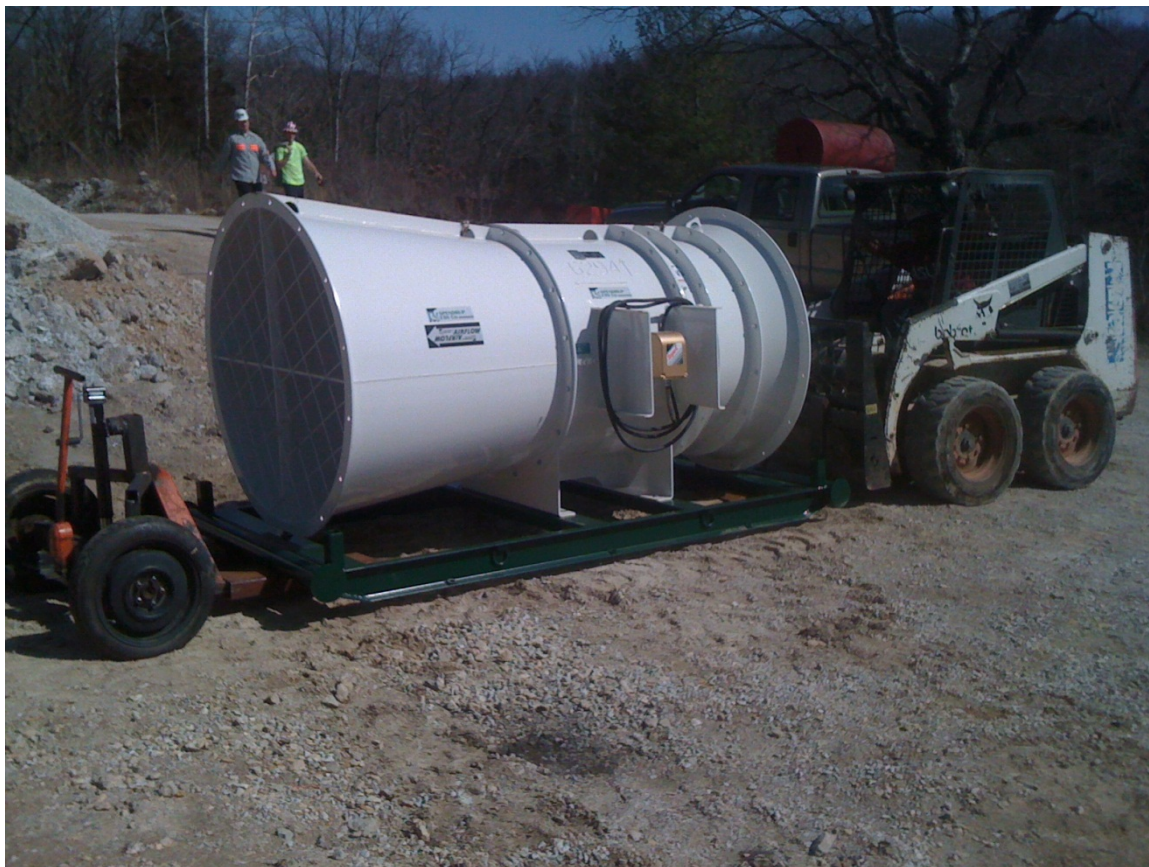
Figure 7.8. Booster fan transportation
