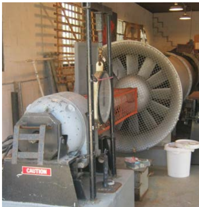
Figure 6.2. Main fan infrastructure at Experimental Mine
